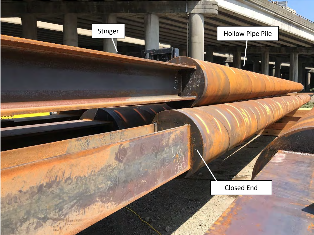
Figure 2: Photo of 24-inch hollow steel piles with H-pile stingers attached at closed end
