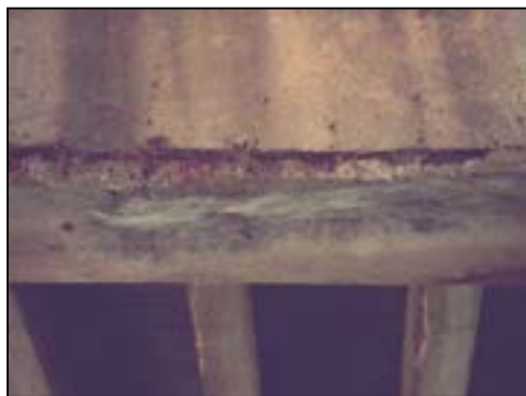
Figure 138. Spall in Pier 2 cap beam. Location 1.
