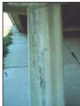
Figure 139. Crack in Pier 3 column. Location 3.
