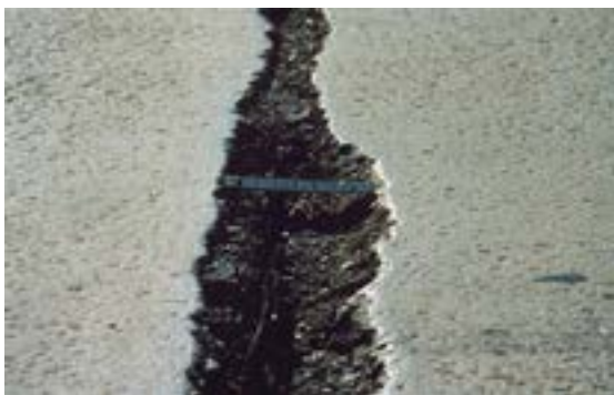
Figure 132. Deck spalling along joint. Location 2.
