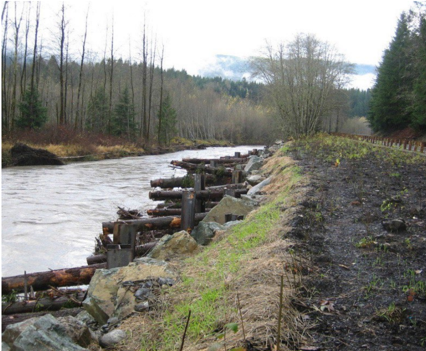
Figure 10A-5 Crib Wall with Steel Piles, Sauk River Side Channel, Skagit County
