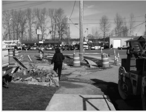
Does not meet ADA requirements
